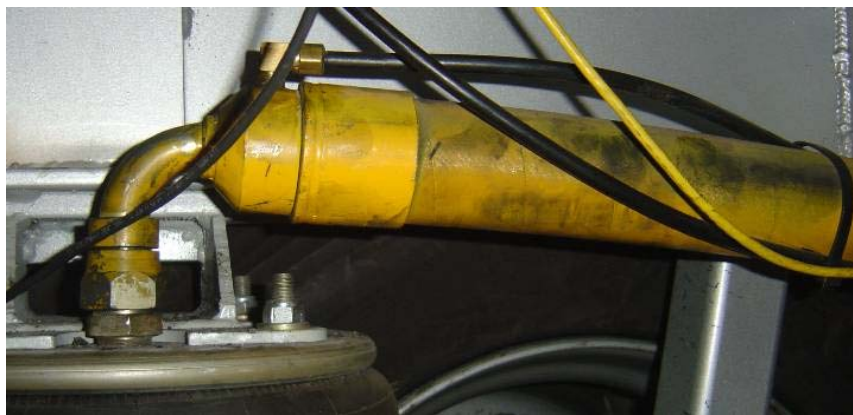
Figure 6 – Large longitudinal air line used in the “Haire suspension system”
