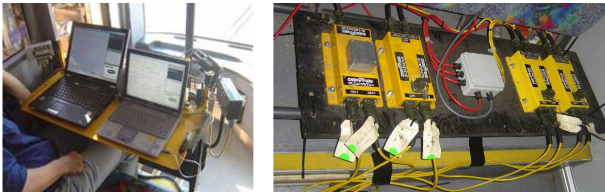
Figure 10 – Data capture management computers (left) and data capture and storage telemetry units (right) installed on a bus
